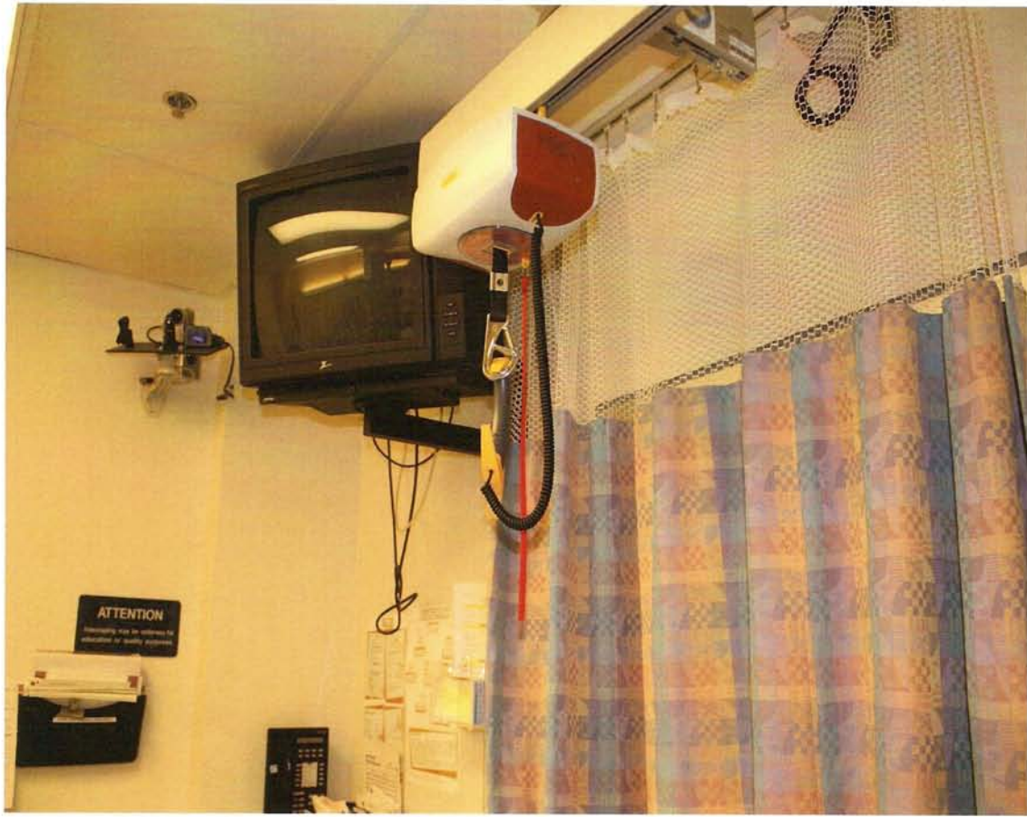
Figure 3: Guldman Overhead Patient Lift System
